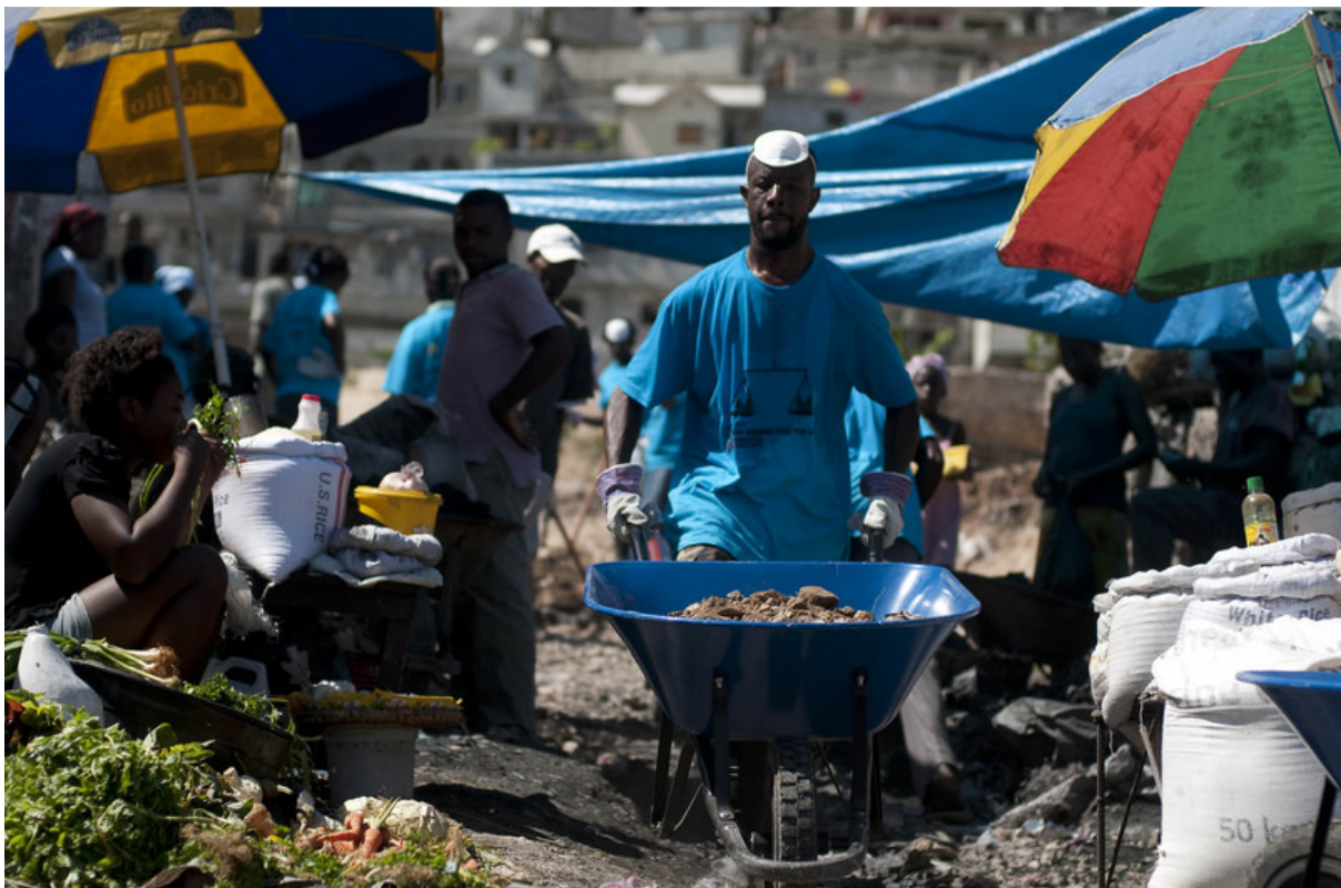
Local residents of Philippeaux, Port-au-Prince take part in cash for work rubble clearing programme sponsored by ActionAid.
